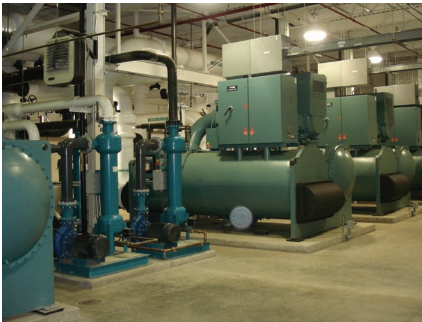
H.T. Lyons provided engineering and construction services for these energy-efficient variable speed chillers at Sanofi Pasteur. Each phase was completed in less than 12 months from design start to final commissioning, according to Craig Kauffman, Manager of Major Project Development.
